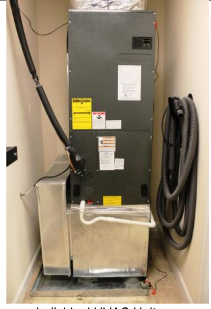
Individual HVAC Units so tenant controls thermostat
