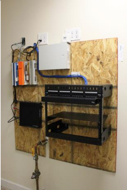
12 pair trunk line from AT&T and coaxial cable from Comcast can easily accommodate any bandwidth need
